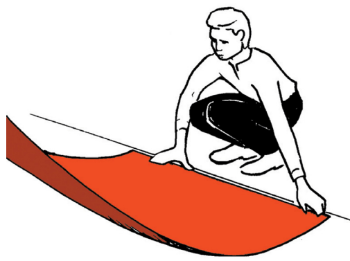
1. Position carefully. Start leading edge with hand before using squeegee, while assistant installer is holding one end up off the ground.
